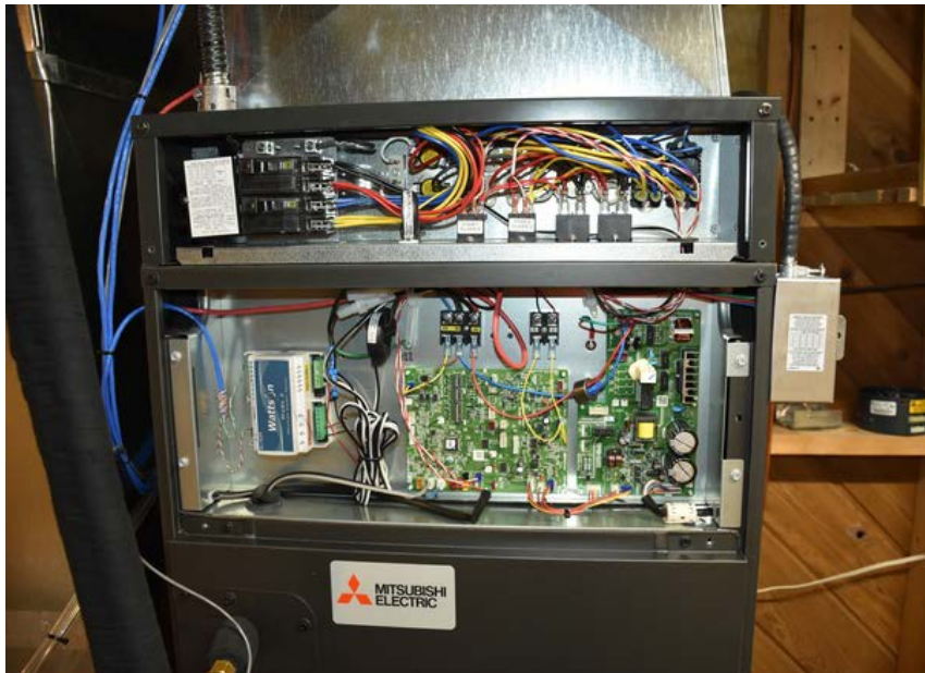
Figure 1: Inside of the indoor cold-climate heat pump unit and the backup auxiliary heat with the power monitoring.
