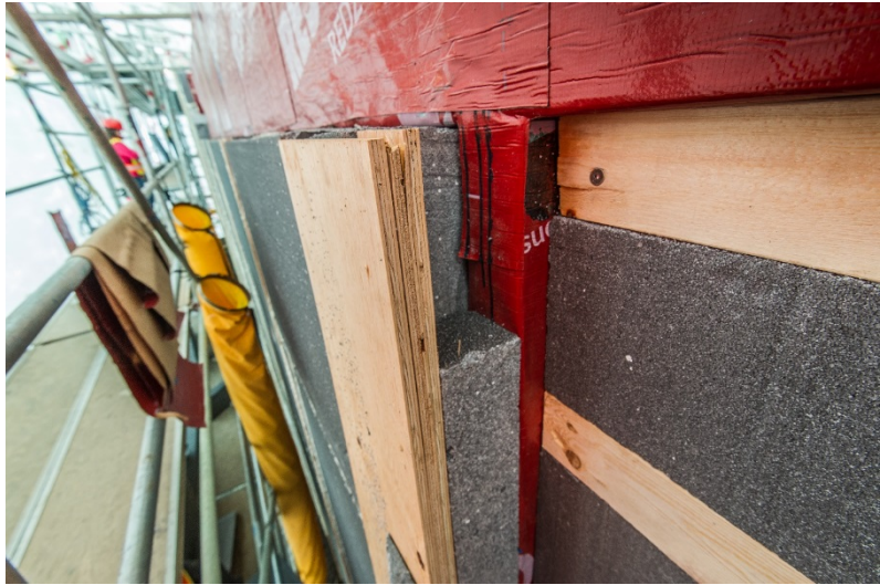
Renovation upgrades, adding exterior insulation to an institutional building. Photo: Government of Yukon.
