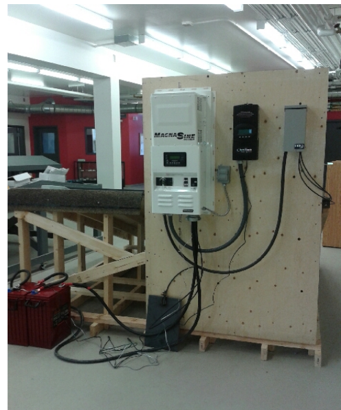
Solar photovoltaic design and installation course where students practiced installing systems. Photo: Government of Yukon.
