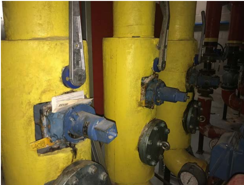
Figure 4: Secondary Pumps' Balancing Valves
