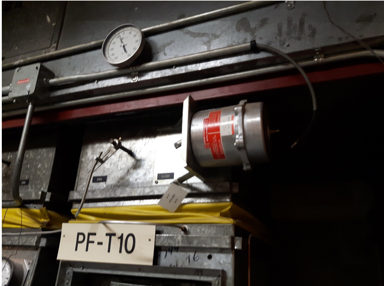
Figure 16: AHU-T6 Damper Actuator
