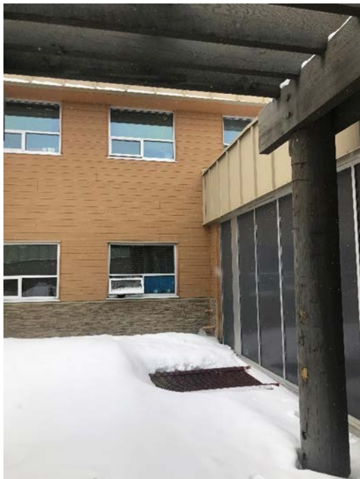
Figure 28: AHU-R1 Outdoor Air Intake
