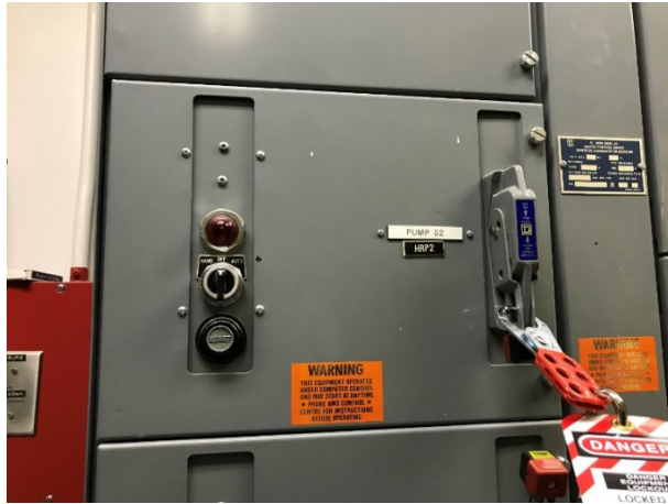
Figure 11: AHU-G1 Heat Recovery Circulation Pump G2 Lockout
