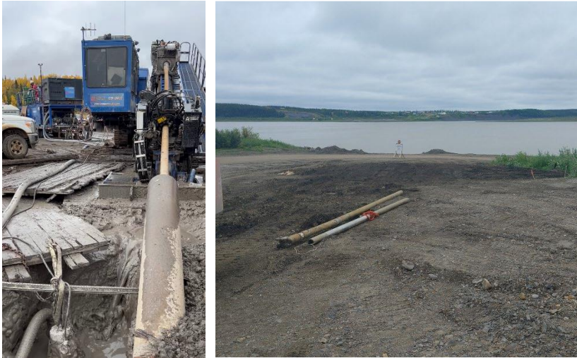
Horizontal directional boring that crosses under the Mackenzie River. The drill exit point on the north bank is pictured on the right.
