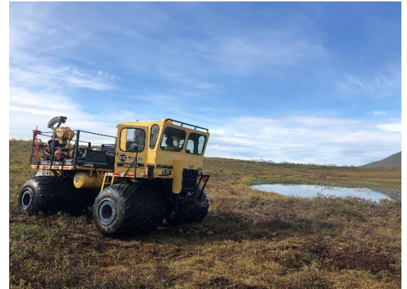
A Rolligon plow vehicle is used to install conduit through tundra habitat. This method minimizes disturbance to the delicate landscape by using low-pressure, balloon-like tires. The pressure of the tires is 15 times less than the pressure a human foot exerts.
