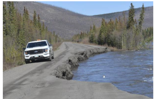
Road washout May 2023
